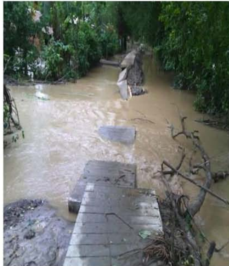
During the Flood
