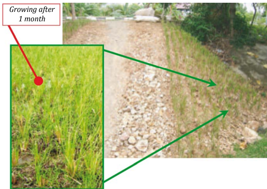
Fast-growing grass was planted on cut and embankment slopes of this road
