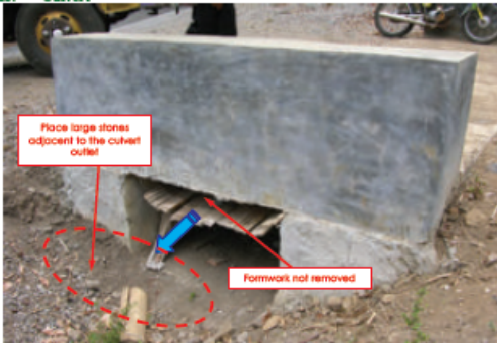
Formwork that is not removed can block the culvert making it useless
