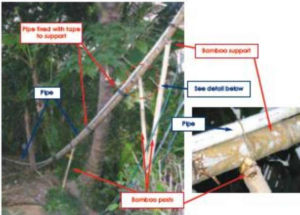
Bamboo support for PVC pipes
