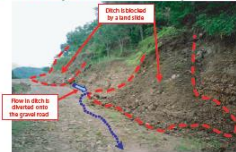
Landslides have blocked the ditch and may soon block the road
