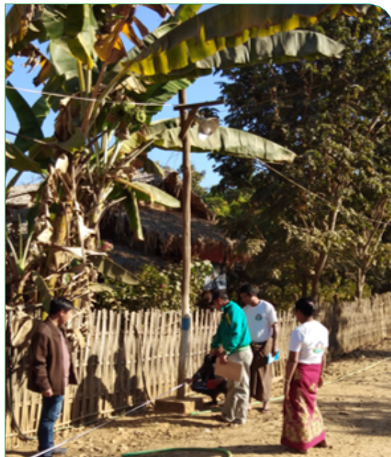
Note: Acceptable locally sourced, peeled electrical conductor support, Bin Ban village, Pi Ti VT, Bilin township
