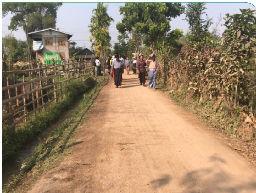
Note: Well-maintained road. Note proper cross-section and camber, clear and open ditch, compact and smooth surface. Khaw Khu (Shan) village, Nan Meh Khon VT, Demorso township.
