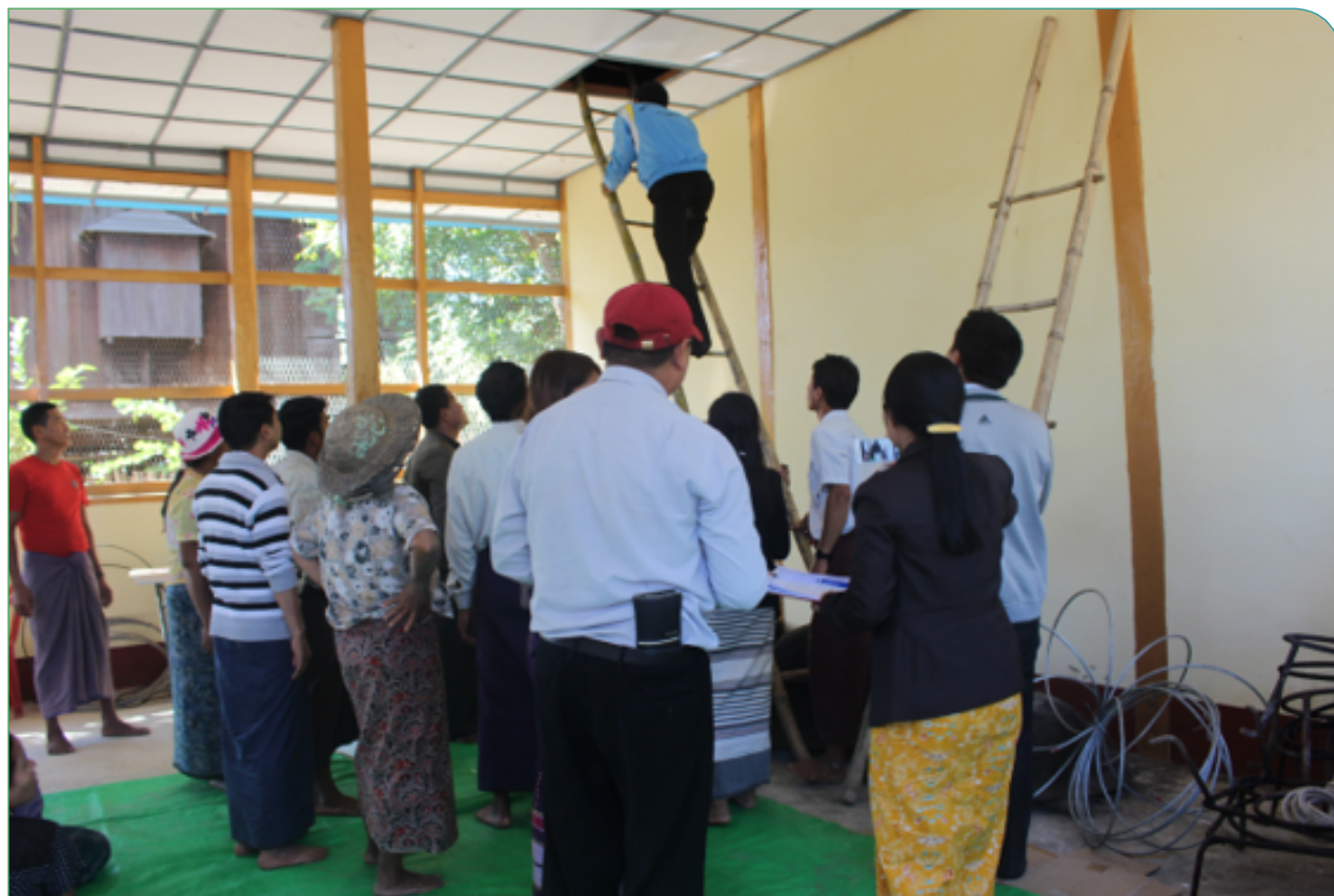
Note: Attic inspection at community center, Nyaung Aing village, Chit Pyin Kaing VT, Sidoktaya township.
