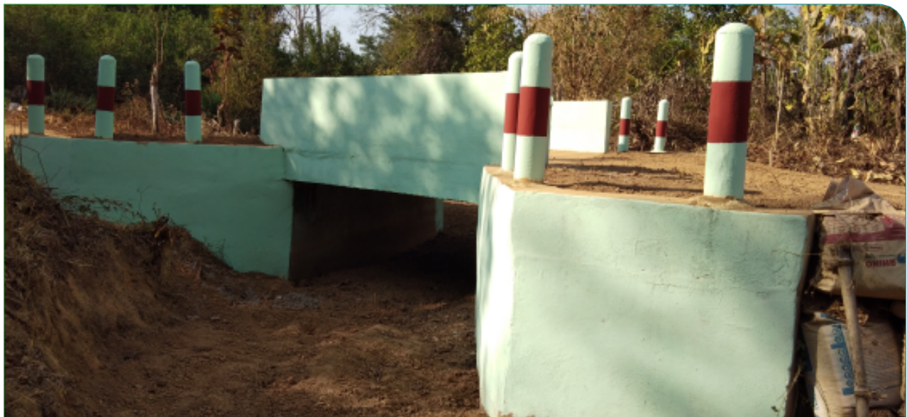
Note: Proper wingwalls. High water flows are controlled and will not erode roadway. Gone Bi village, Nat Ghaung Kannar VT, Kyarinseikgyi township.
