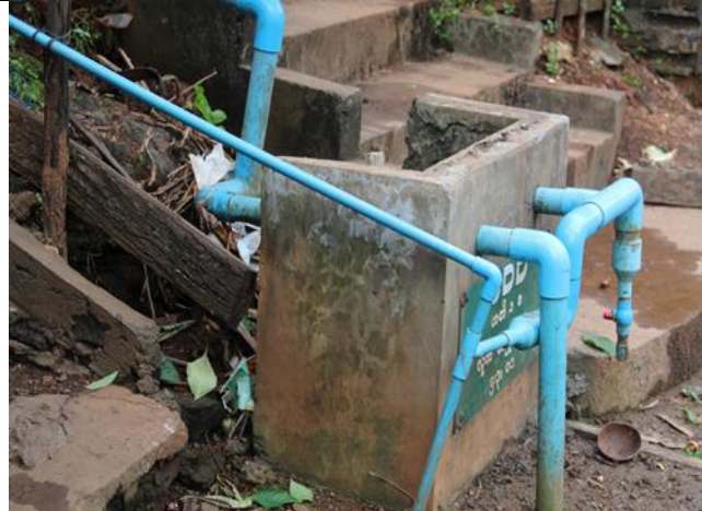
The piping installation system need proper fixing system (to avoid damages) Ma San Par village
