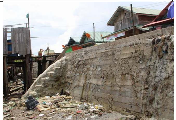
Pa Htaw Village , Constructed stone masonry Retaining wall at river side to prevent erosion, which damaged and lost for the village,
