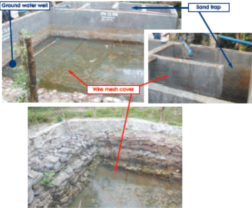
Wire mesh protection over a ground water well
