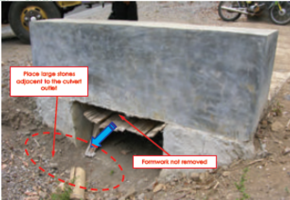
Formwork that is not removed can block the culvert making it useless
